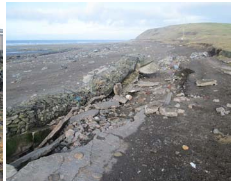
Damage to concrete plinth and gabion baskets at Parton. Due to access problems it was only possible to undertake a mass concrete pour to stabilise the area.
