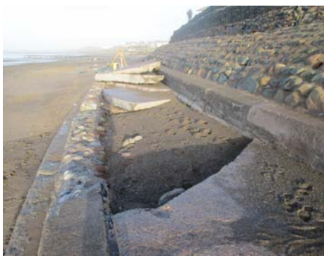
Seascale Seawall - Part of the concrete slab was ripped off during the storm on 3 rd January. This is a Cumbria Highways structures and has been repaired. The surveyors are checking for movement in the bank behind the structure.
