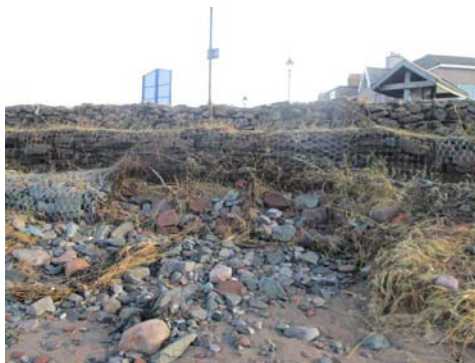
Damaged gabion baskets at Seascale. Rock armour has now been placed in front of these for protection.
